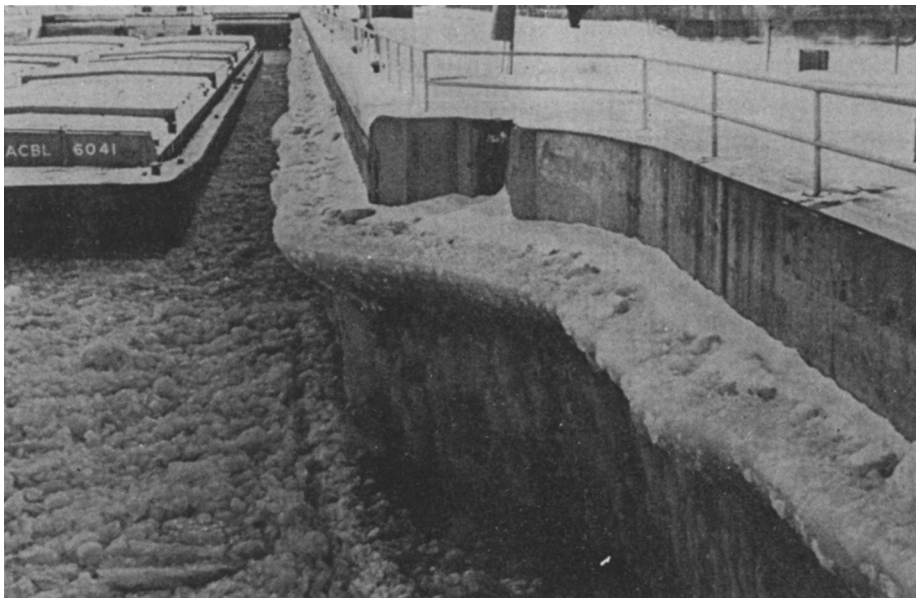
Figure 3-4. Ice collar formation on the gate recess and chamber walls, restricting the full opening of the miter gates and limiting the usable width of the lock.
